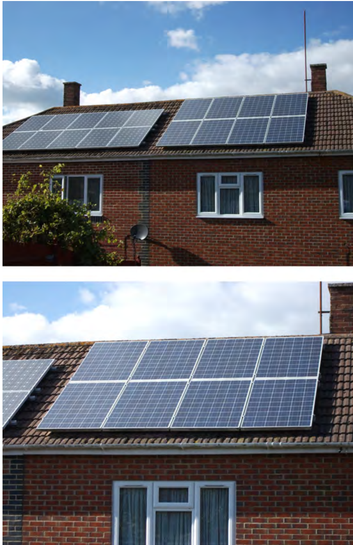
Figure 7.2. Domestic solar panel installations in the UK. (a) Adjoining properties with solar panels fixed to south facing roofs. (b) Closer view of an 8-panel 1 920 kwh (per year) rated system with the panels wired in series, installed circa 2011. (Images © Dave Culpeck. Reproduced with permission.)
