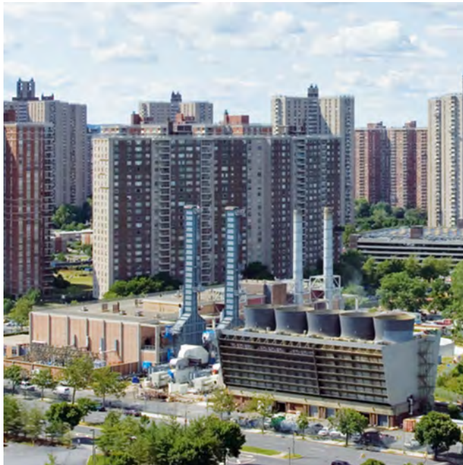
Figure 2.4. The combined cycle power plant at Riverbay Co-Op City in New York, USA. (Courtesy of Siemens. © Andreas Messner. Reproduced with permission. www.siemens.com/press )
