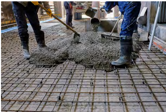
Figure 2.16. Creating reinforced concrete by pouring concrete over steel rods. Concrete itself is also a composite material, comprising a mixture of sand, cement, an aggregate such as gravel or crushed stones, and water. (© seroma72/Shutterstock.com).
