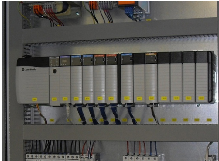
Figure 1.5 – An Allen-Bradley rack-mounted PLC
